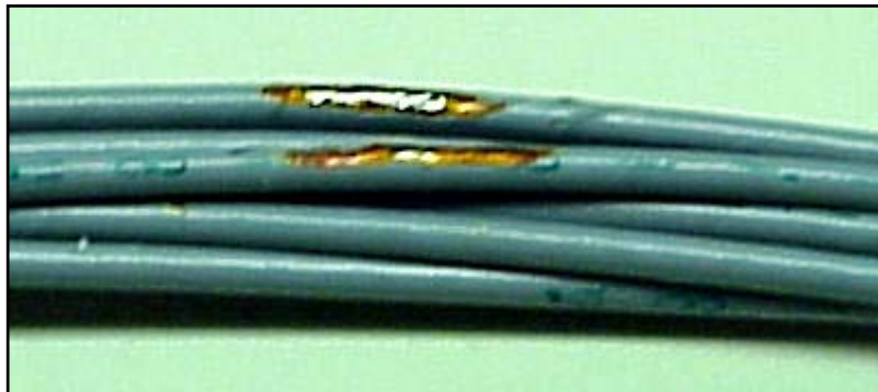
Damaged wires prone to arc over
