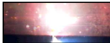
High Level Arcing (>100 Amps) After Flashover
